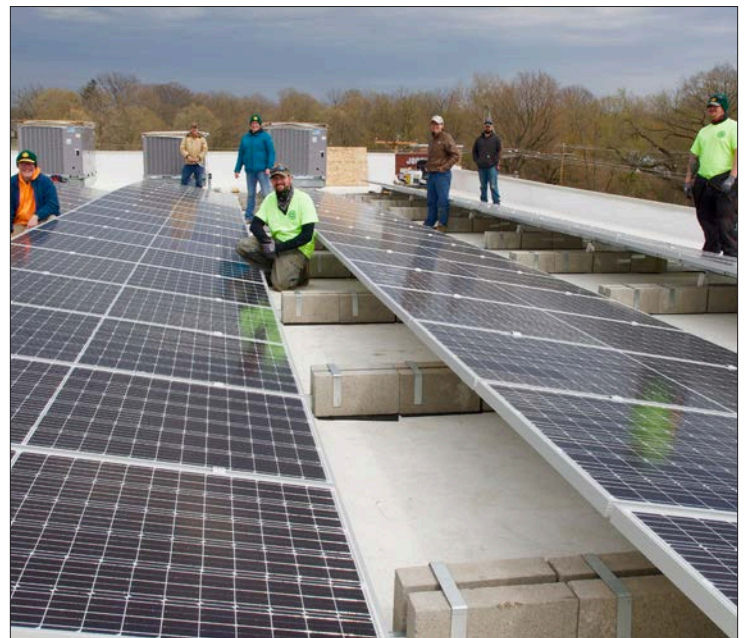
Solar energy system on REES roof.
